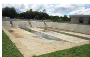
Low Lift Pump station and Sludge Drying Beds
